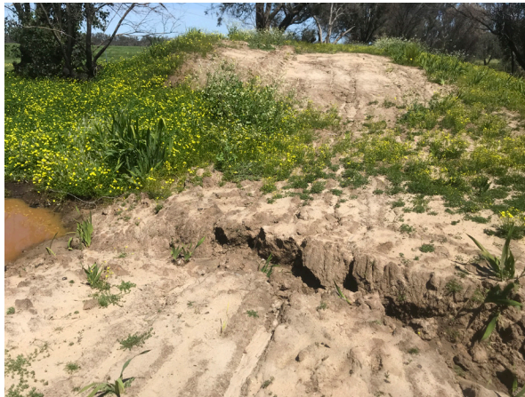
Figure 20: The ephemeral drainage line entering the Birrega Drain site. Top photo is looking upstream along the bank of Birrega Drain (note the erosion from the drainage line in foreground). Bottom photo is taken from the same spot looking upstream along the drainage line in September 2020.
